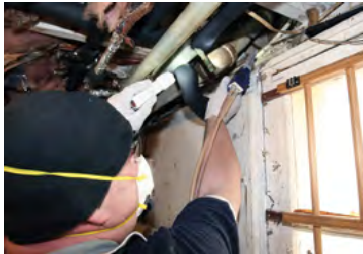
Crew member seals air leaks in a basement. Photo: ©2012: Advantage Weatherization, Inc.
